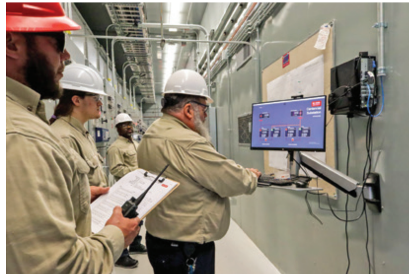
Top: An NC State line technician operates a switch at the new substation on Centennial Campus. Bottom: Connecting parts of the new system into the university’s SCADA system enables the team to receive alerts and find problems before they become outages. Photos: Matthew Wright, courtesy of NC State
